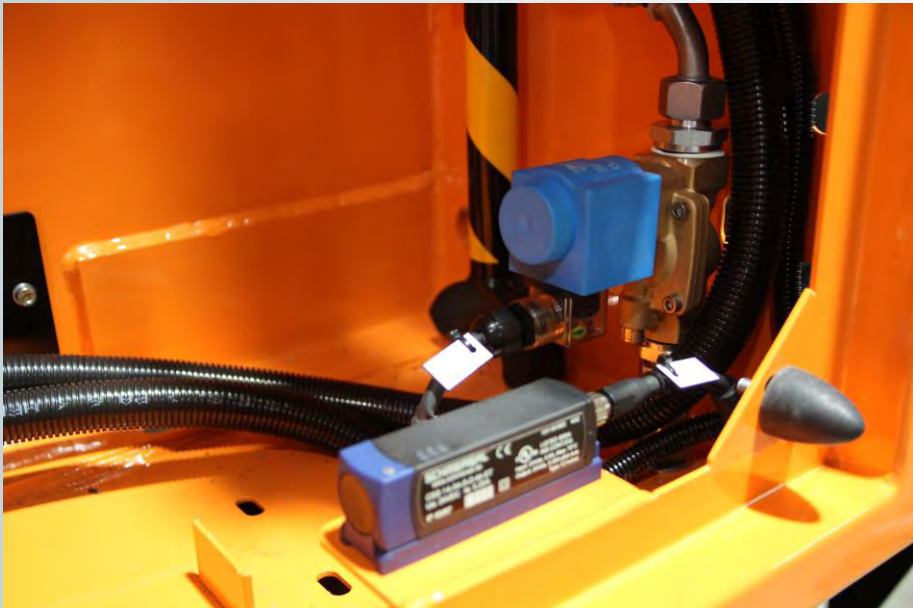
Security sensor CSS34, without guard locking, example: door for distribution box
